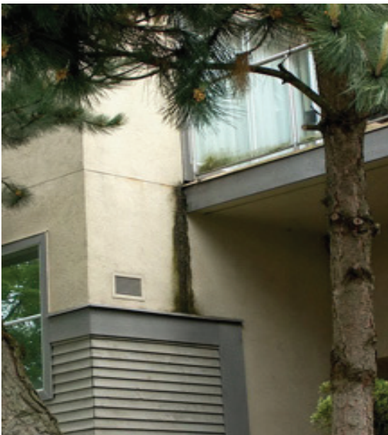
Concentrated balcony runoff leads to an unsightly appearance and potentially premature failure of the wall if not addressed
